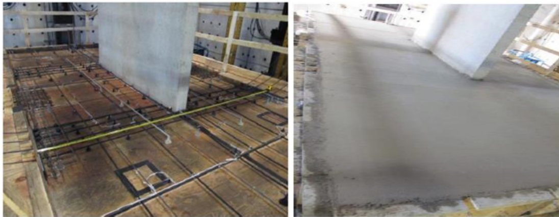
Figure 13 Layout of the reinforcement and strands of the floor slab before and after casting of the specimen (Liu 2016).
