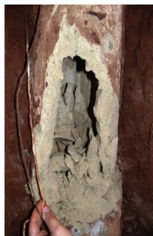
Figure 14 Another detail of the defect after load tests performed on DPR_{(EXP)} system.
