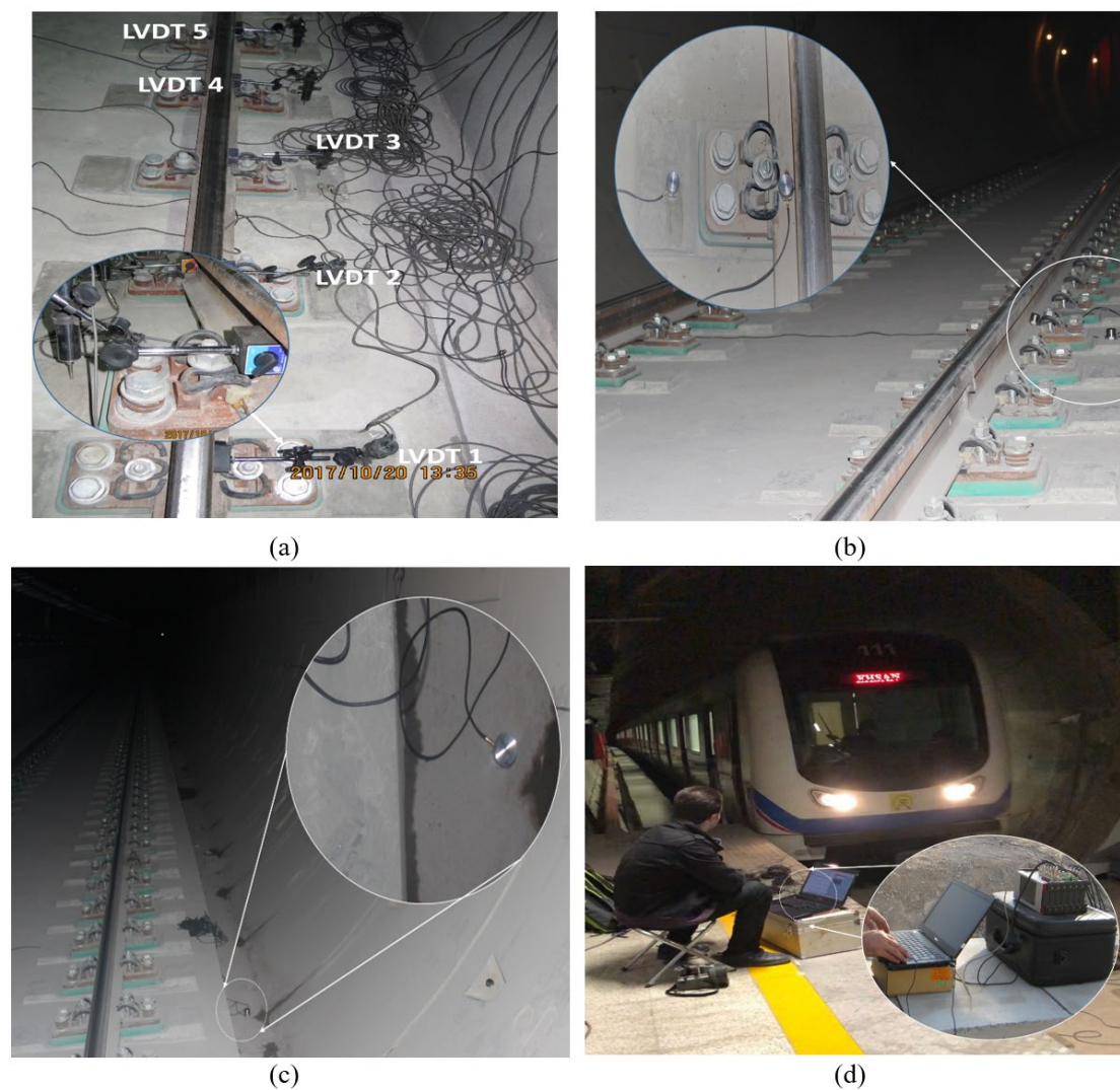
Fig. 5. Field measurement (a) LVDTs installed for track stiffness measurement, (b) Installation of vibration sensors (accelerometers) on the slab, (c) Installation of vibration sensors (accelerometers) on the tunnel base, (d) Data logger and laptop computer used for the measurement at each train pass
